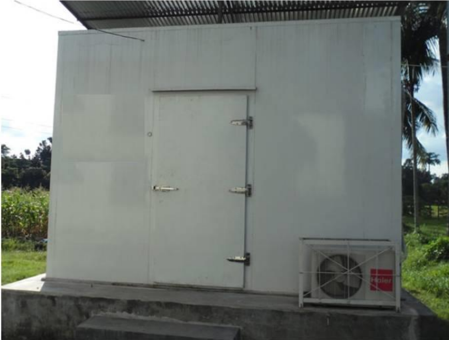
Photograph 3: A coolbot in use in Bangladesh
